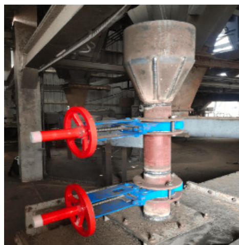
Figure 10 Feeding system for Oxy-booster
