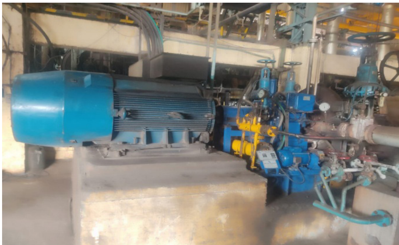
Figure 8 Back Pressure Turbine
