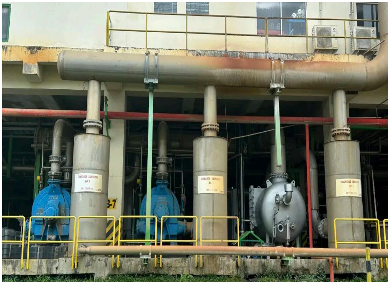
Figure 6 Installed CIGU maglev turbine vacuum pumps at APP Indonesia
