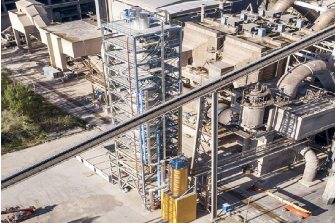
Figure 11: LEILAC direct separation technology illustrating indirect calcination and its integration within a cement plant for process CO 2 capture
