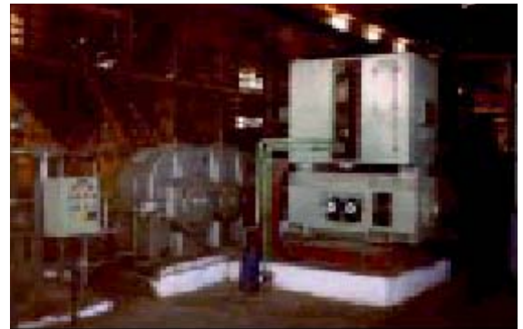
Electric DC drive for mill
