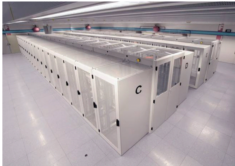
Typical installation of cold air containment
